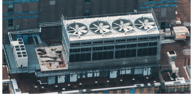
Figure 1: Four Cooling Tower Fans
