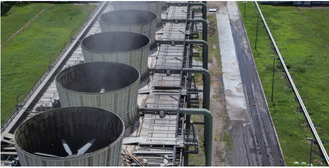
Figure 5: Cooling Tower Fans
