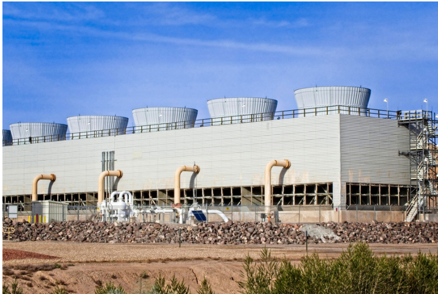
Figure 6: Cooling Tower with Five Fans
